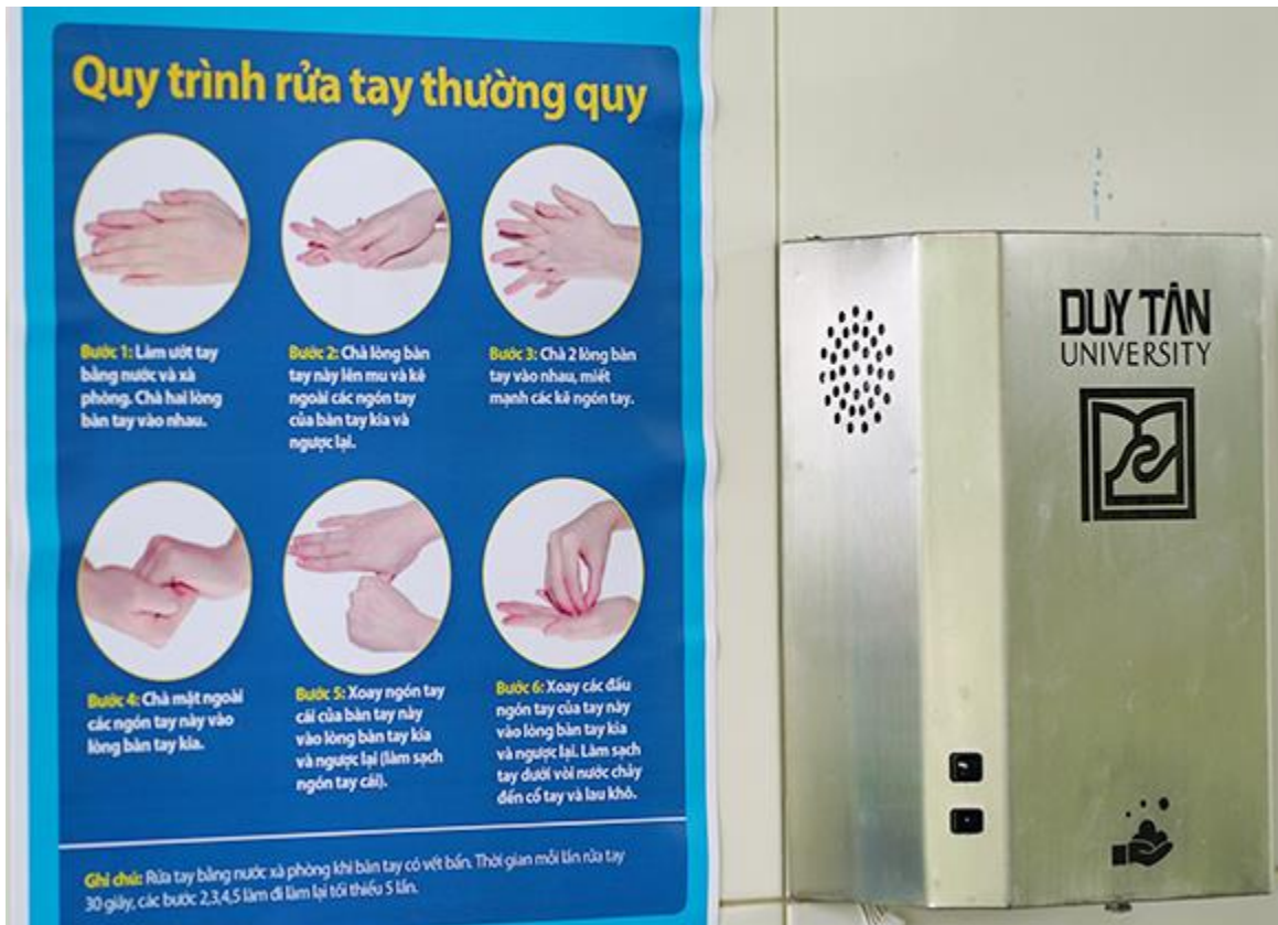
Hand washing instruction device installed at DTU
